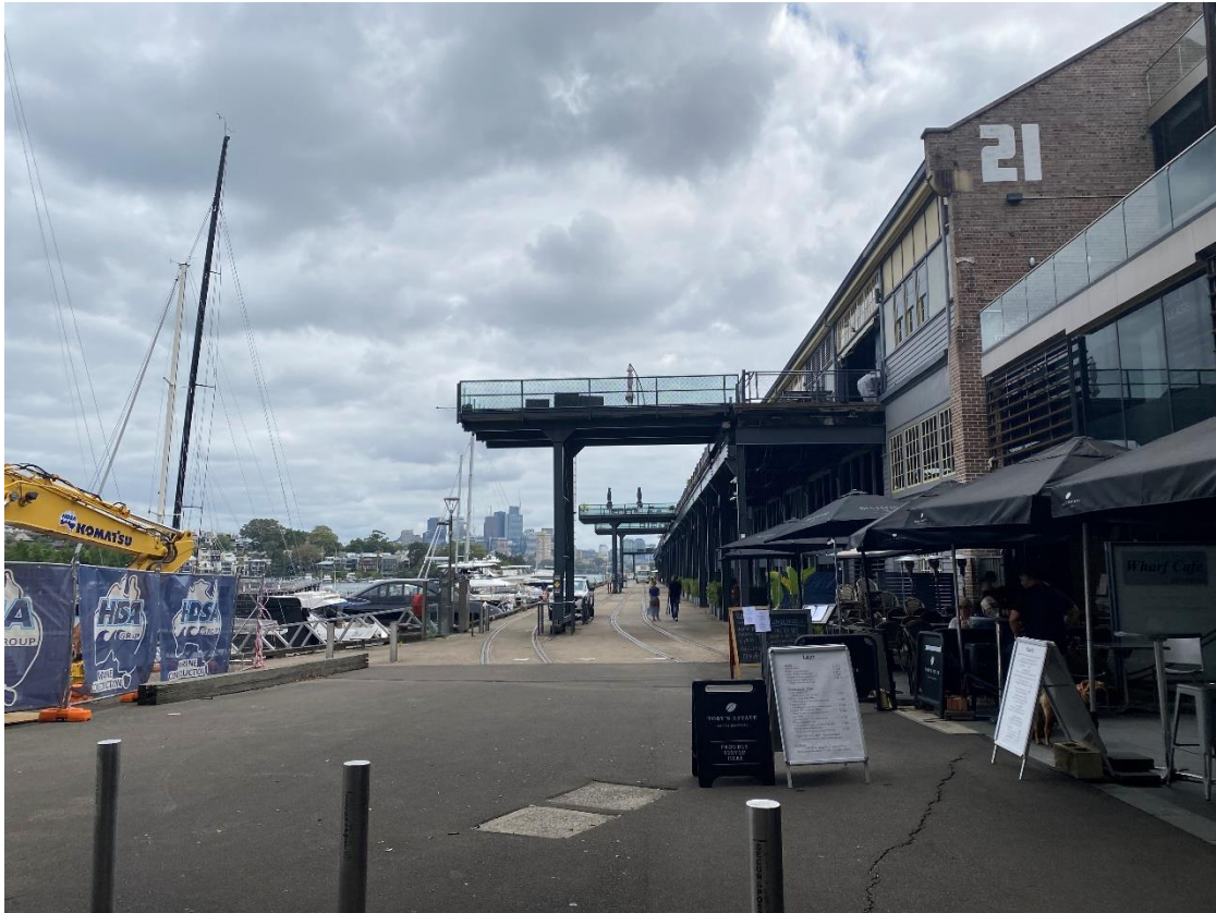
Figure 7: Site viewed from Pirrama Road, looking along the western side of the wharf
